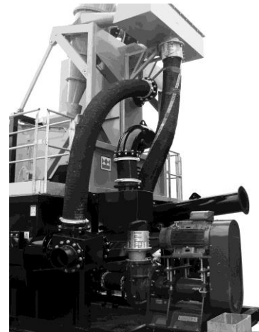
Rubber lined sealed slurry transfer pipes complete with heavy duty clamps
