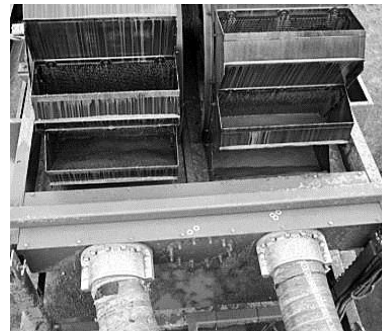
Anti-turbulence inlets in bucket tank
